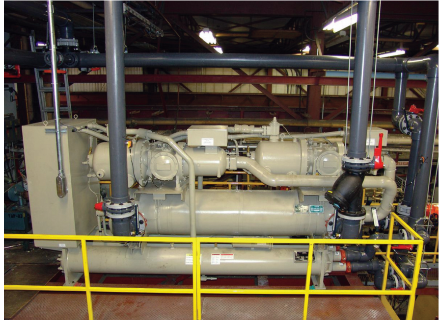
The McQuay water-cooled screw compressor Model WGS Chiller installed at the Camoplast automotive component injection molding facility is part of the energy award winning system that reduced annual energy costs by 70%.
